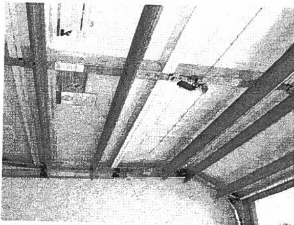
Garage doors are reinforced and wind rated.
